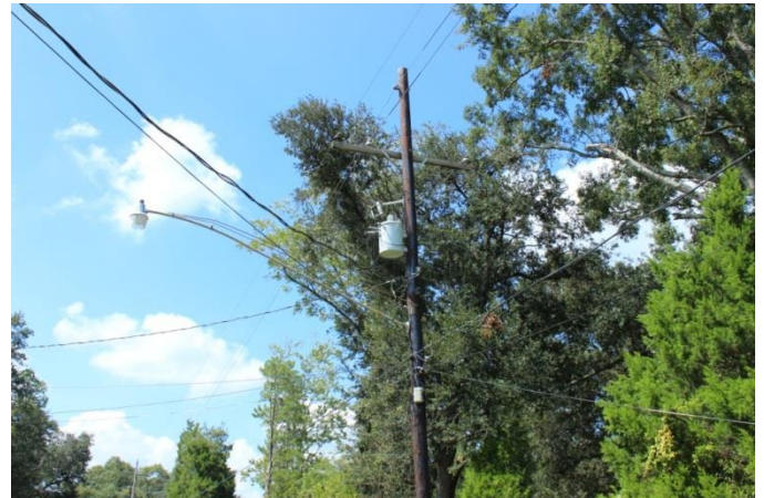
Replaced transformer a block away which was the location of the problem.
